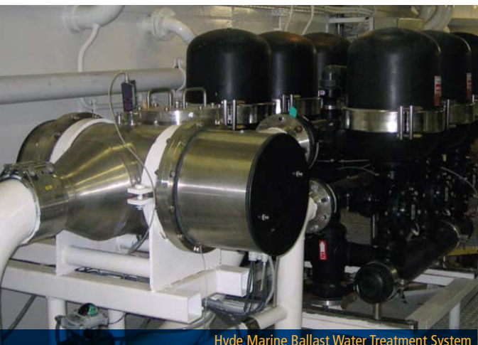
Hyde Marine Ballast Water Treatment System
